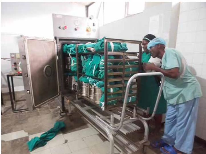
Fig. 5: Loading one of the two autoclaves based on the AmSCO Medallion at the Bugando Medical Centre, Tanzania (29.11.2019).
