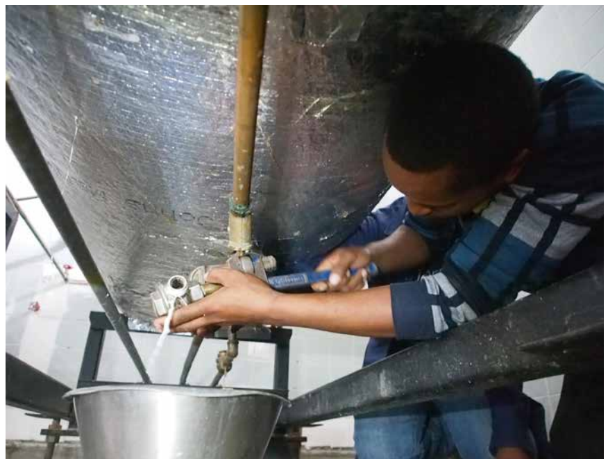
Fig. 8: A technician removes the steam trap that turned out to be defective (04.12.2019).
